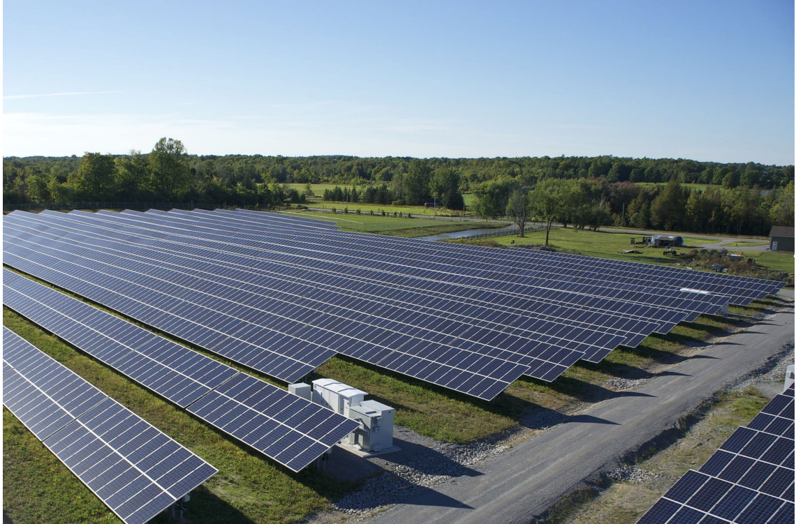
Figure 4.2: Typical Fixed Panels (with Conversion Unit / Inverter)
