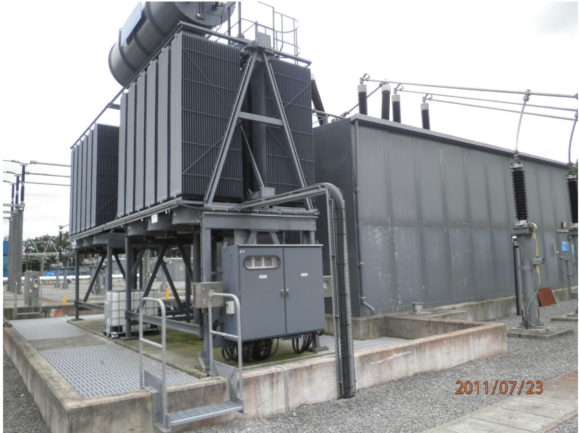
Figure 4.3: Typical (large 400kV) power transformer
